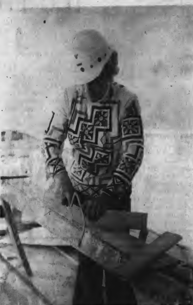
A coping saw is used to trim a base board to fit into a corner. Once she has completed her inspections, Mrs. Bercaw helps do the work on the job.
